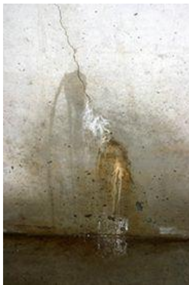
Groundwater can cause soil to crack foundations
