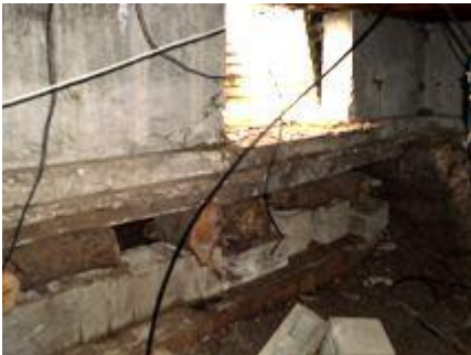
In this picture, an inspector found a homeowner was shoring up their foundation with logs
