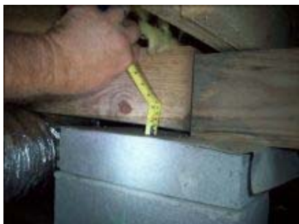
Sloping Floors caused by sagging girders and floor joists.
